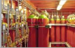
Gas firefighting system
